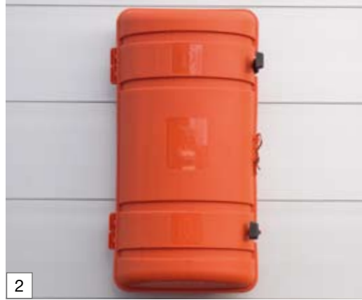
2 Fire extinguisher fitted on the bulkhead
